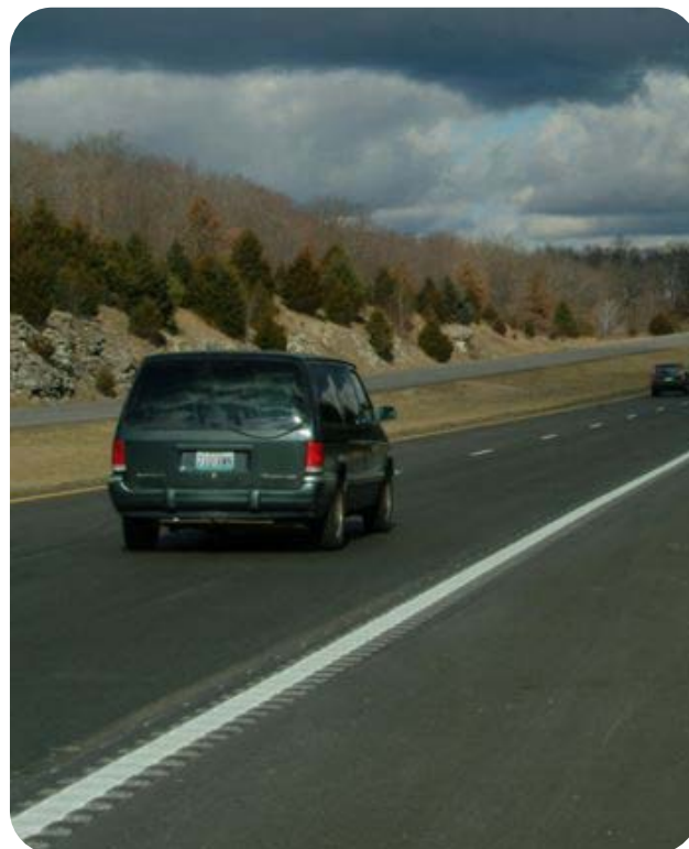
Edgeline Rumble Strips
